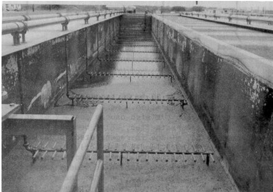
Figure 2-19. Aeration tank with diffuser tubes.
